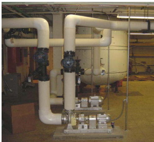
Fig 8: Circulation Pumps and Storage Tank
