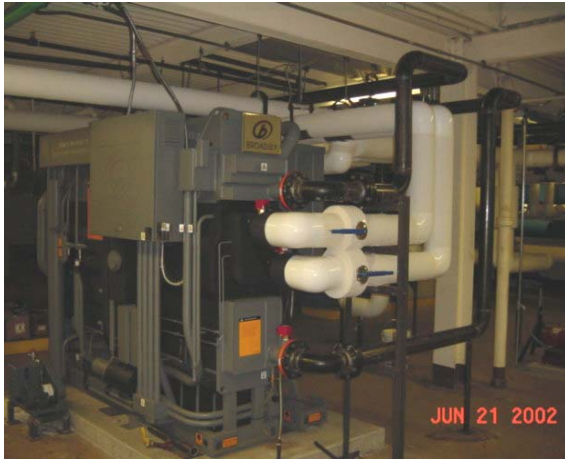
Fig 7: 50-ton Double-Effect Absorption Chiller
