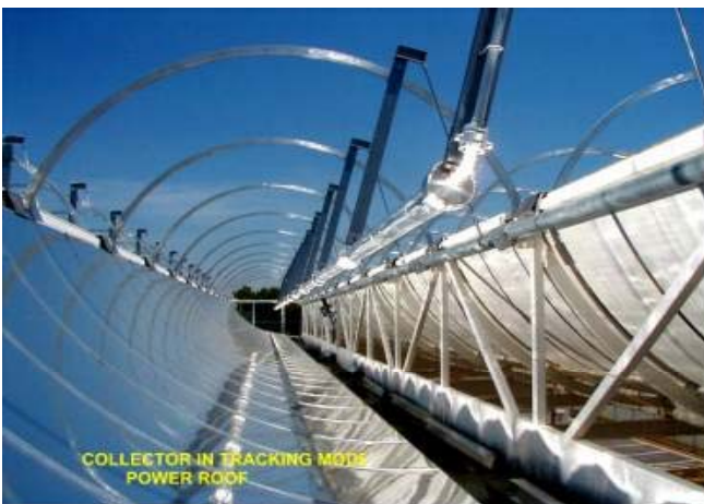
Fig 1: Power Roof™ Installed in Raleigh, NC
